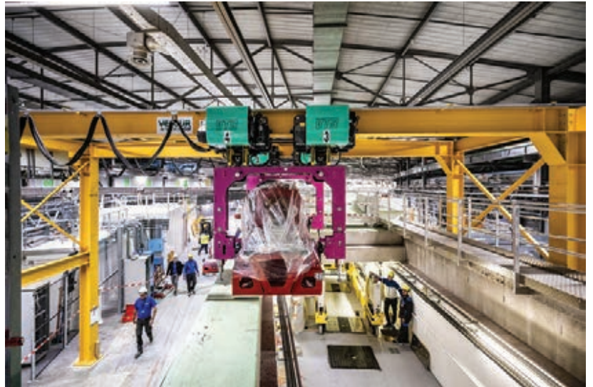
Fig. 3: The impressive installation of 129 pre-assembled girders in the storage ring tunnel started in March 2019.
