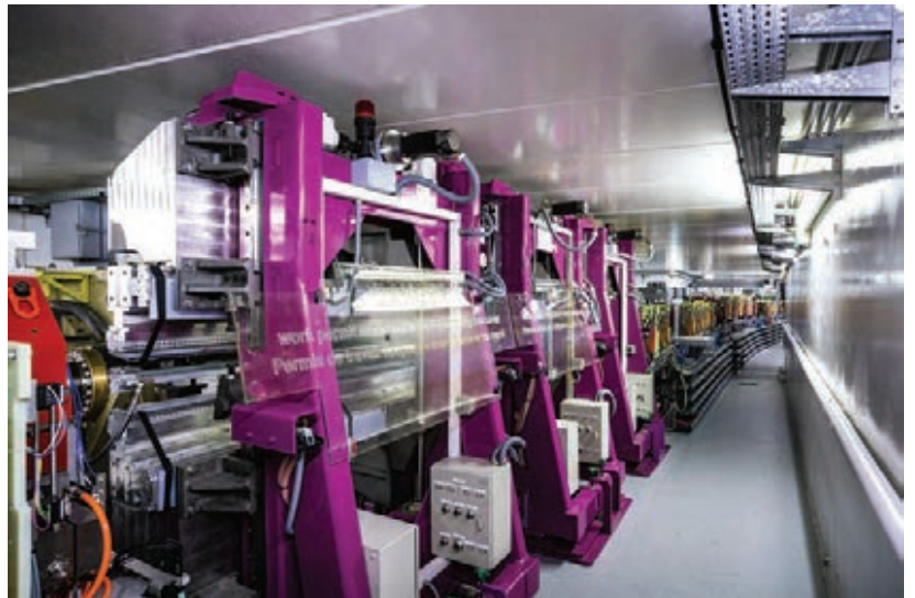
Fig. 4: Following the completion of the girder installation in May, the insertion devices were installed in the storage ring tunnel from July to November.
