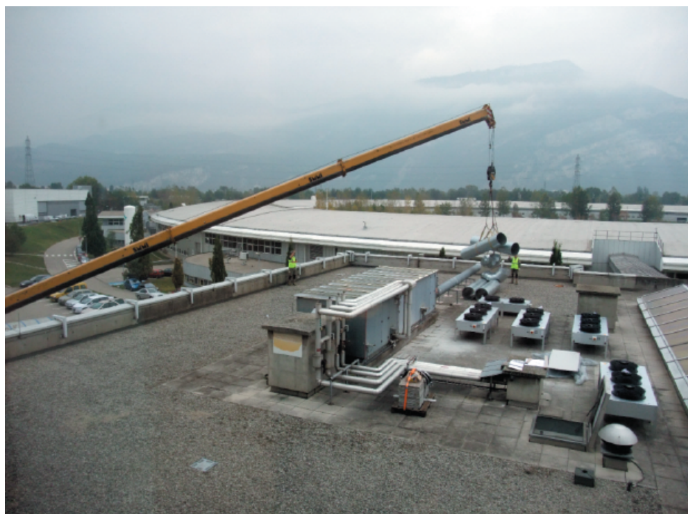
Fig. 151: Installation of the heat exchangers on the roof of the ESRF central building.
